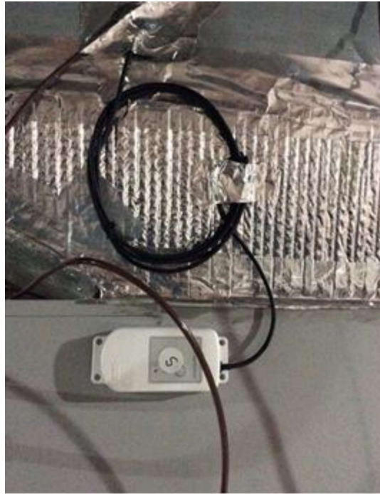
Figure 2-6. Example of Central Heat Pump Supply Air Temperature Logger Installation
