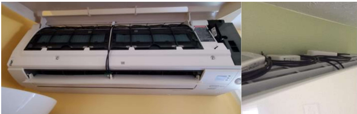
Figure 2-8. Example of Mini Split Heat Pump Indoor Unit Logger Installation
